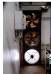
Figure 3. Forced ventilation fans
